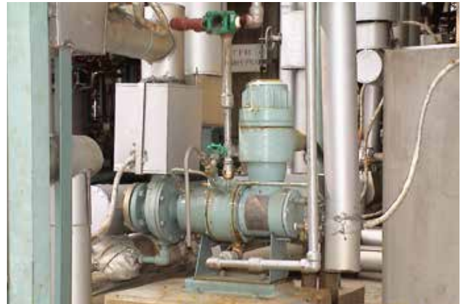
High-temperature type pump in a chemical plant.
