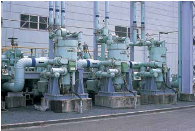
Reverse circulation type pumps for pumping LNG as Cooling medium. (Vertical type, Motor output 75kw)
