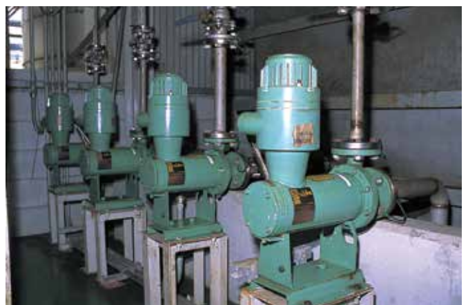
Basic type pumps in a chemical plant.
